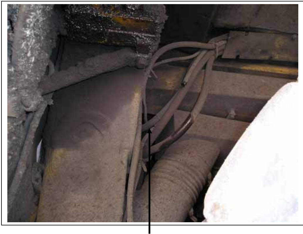
Hoses from cab running over to left side of engine.
